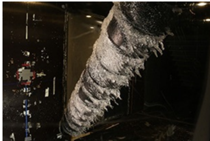
(b) Ice accretion on bridge cable
